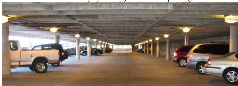
...leaves this municipal deck in downtown Erie, PA lightly uses on most days
